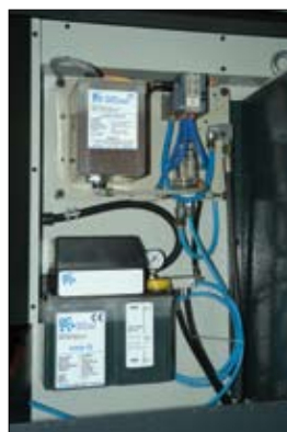
Lubricating system cabinet
